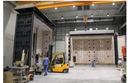
Fig. 1 Installation of the 5 m x 5 m furnace in the ift Fire Safety Centre
